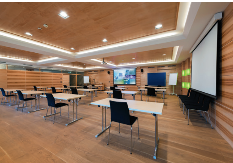
A DXP HD 4K matrix switcher installed in a central control room can support two or more adjacent classrooms.
